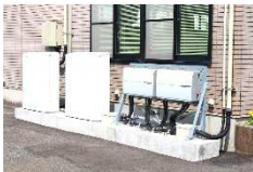
蓄電池15.6kWh (7.8kWh×2)
